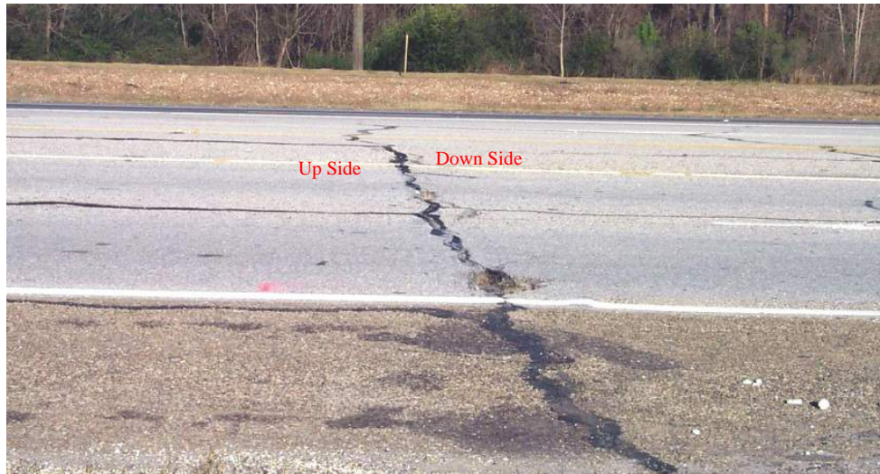
Figure 64 – Recent Crack along GPR Profile 4: Willow Creek Area Likely Caused by Dislocations Shown in Figure 62 as Profile 4b. Looking East across the Highway.
