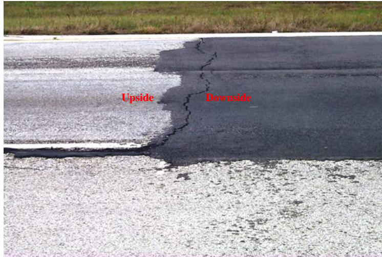
Figure 55 – GPR Profile 1: Iowa Colony Site Looking West across the Northbound Lane (2005) (Note recent patch with more recent crack)
